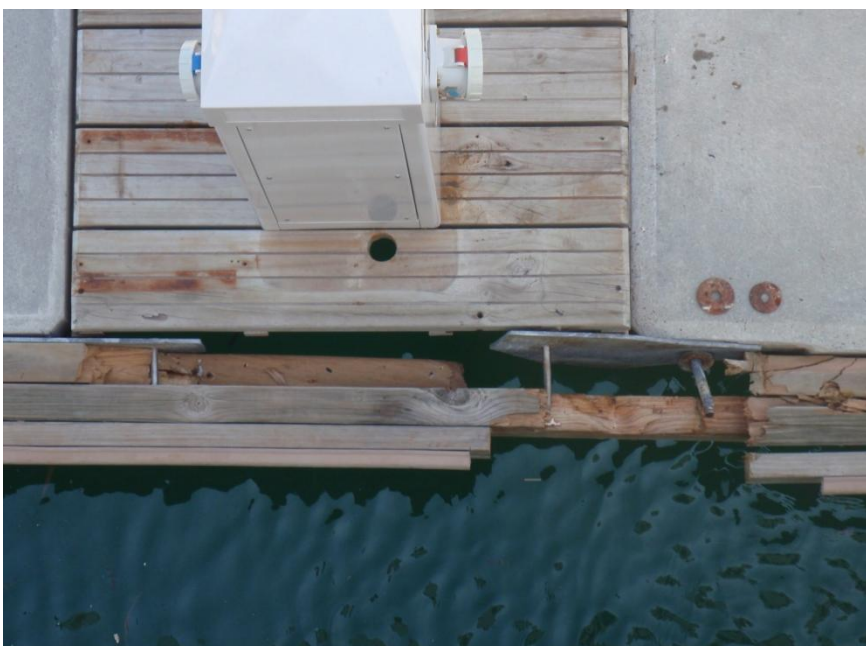
Figure 14: Failed bollard mounting through one concrete pontoon and one backing plate.
