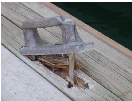
Figure 10: Failed Stern Cleat
