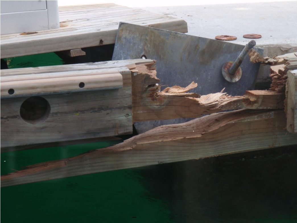
Figure 20: Damage to quayside
