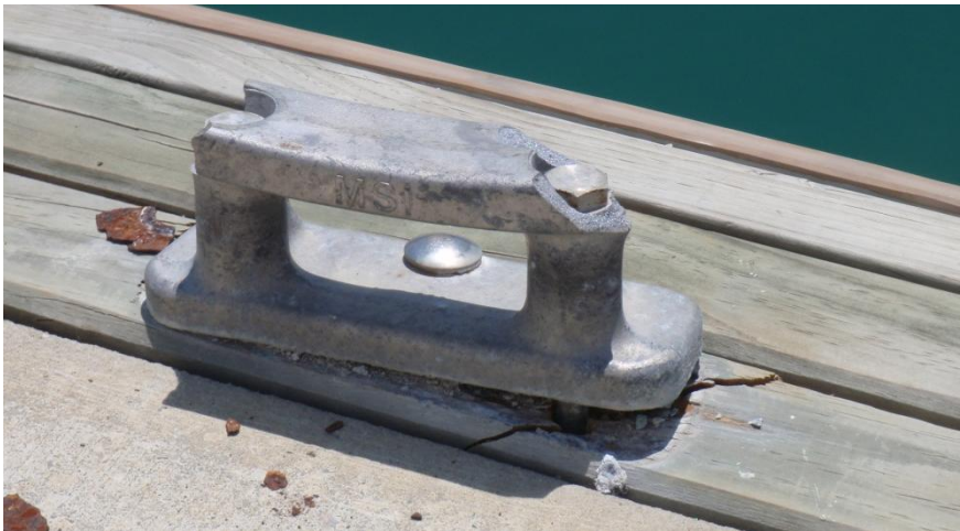
Figure 11: Failed headline cleat
