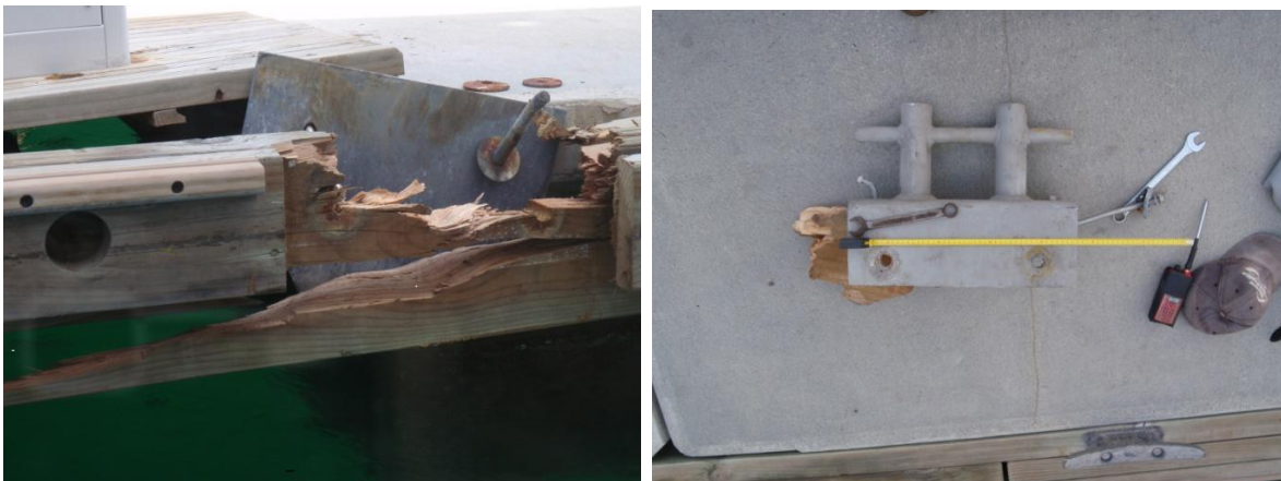
Figure 12: Bollard pulled from quay
