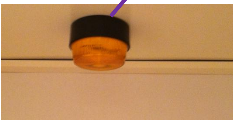
Visual Alarm (Door Closing)
