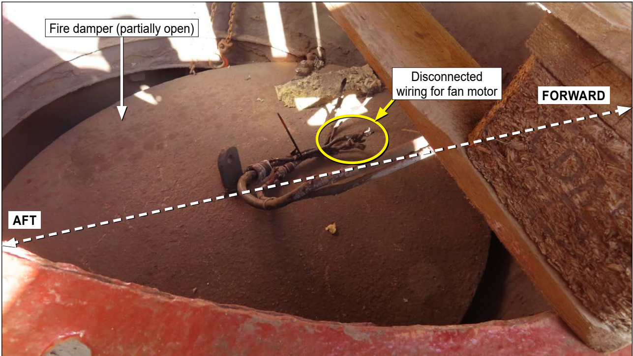
Figure 4: Starboard engine room fan pedestal fire damper
