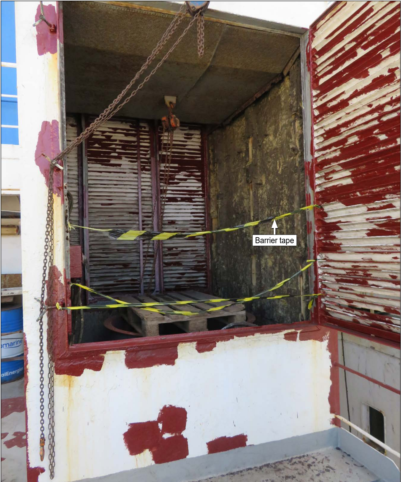
Figure 9: Barrier tape across the fan room access
