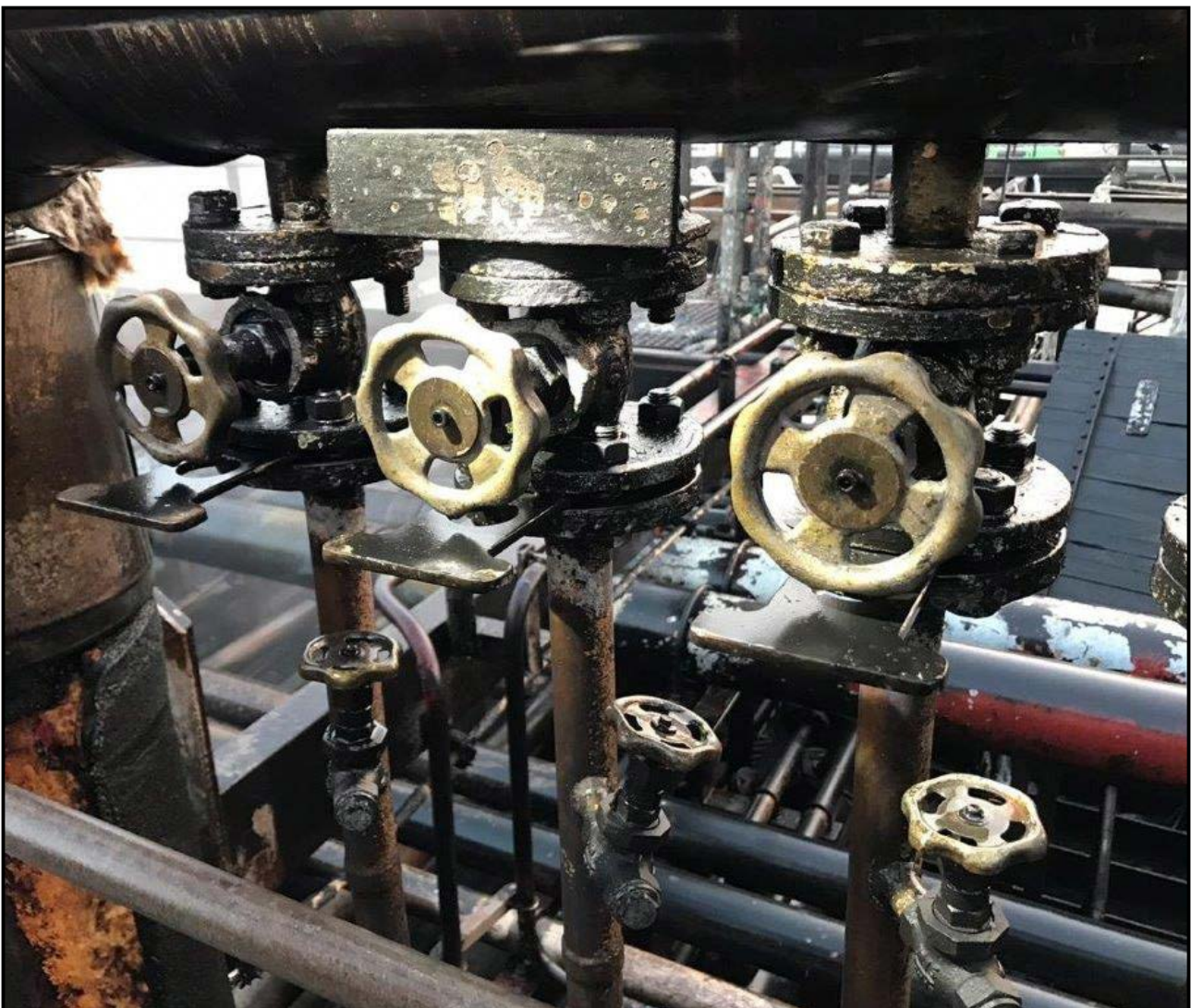
Figure 10: 9S heating control valves
